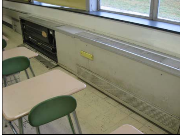
Typical Classroom Unit Ventilator
