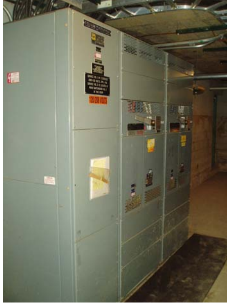
Figure E-1. Service Entrance Equipment One
