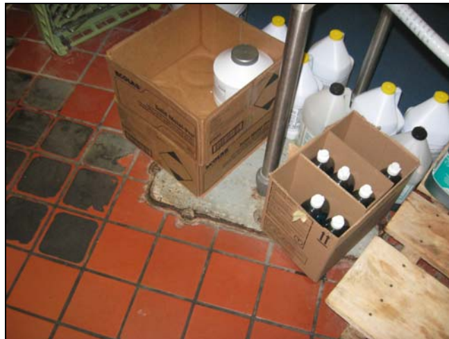
Grease Interceptor in Kitchen Floor
