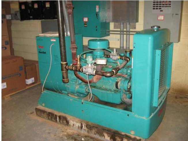
Figure E-4. Indoor Emergency Generator
