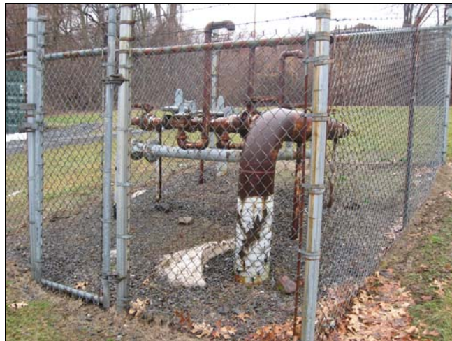
Main Natural Gas Service Entrance
