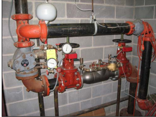
Sprinkler Water Service Entrance
