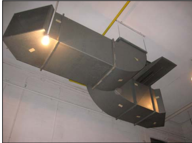
Combustion Air Ductwork at Boiler Room Ceiling
