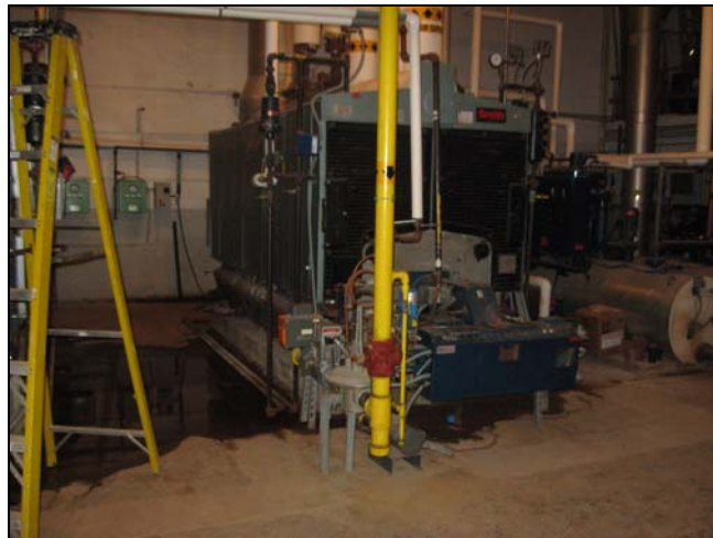
One of Two Steam Generating Cast Iron Sectional Boilers
