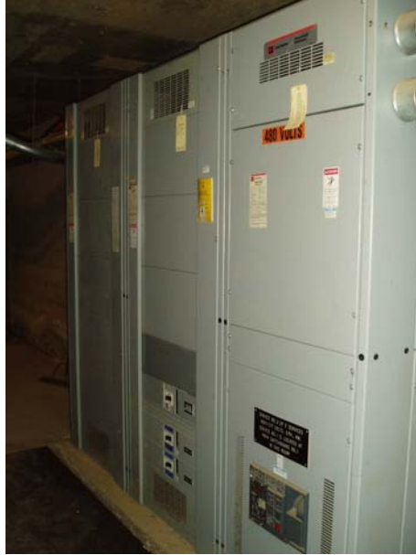
Figure E-3. Service Entrance Equipment Two
