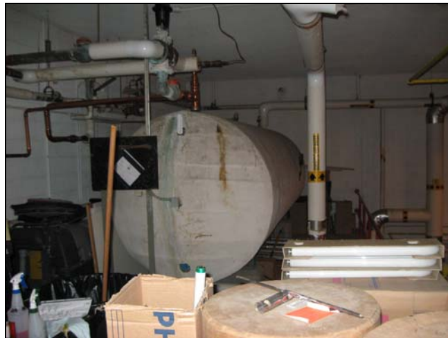
Domestic Hot Water Storage Tank
