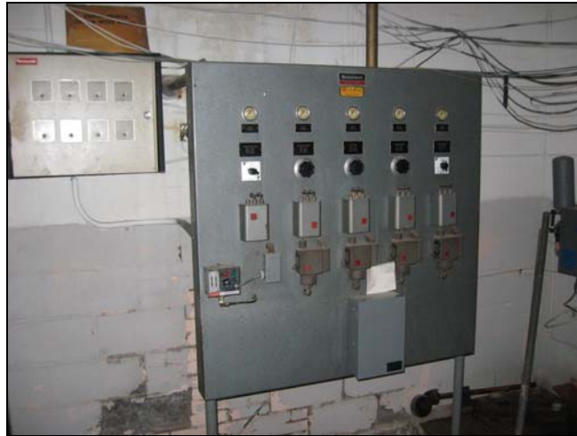
Pneumatic Control Station
