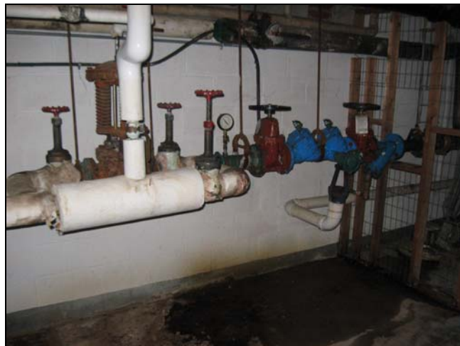
Water Service Entrance
