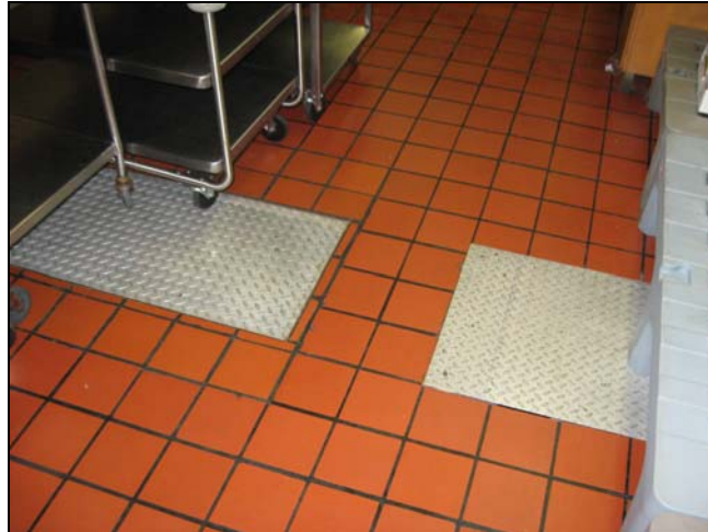
Grease Interceptors in Kitchen Floor
