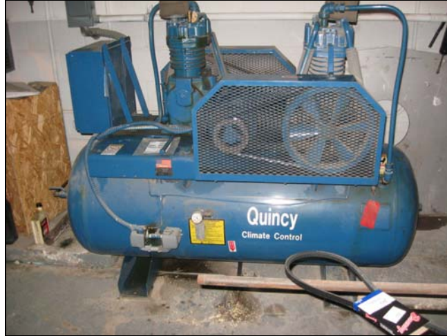
Air Compressor for Operation of Pneumatic Control System
