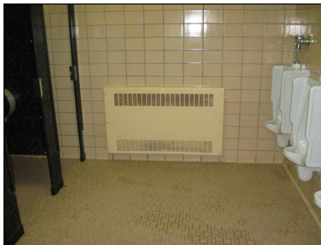
Heating Convectors in Typical Toilet Room
