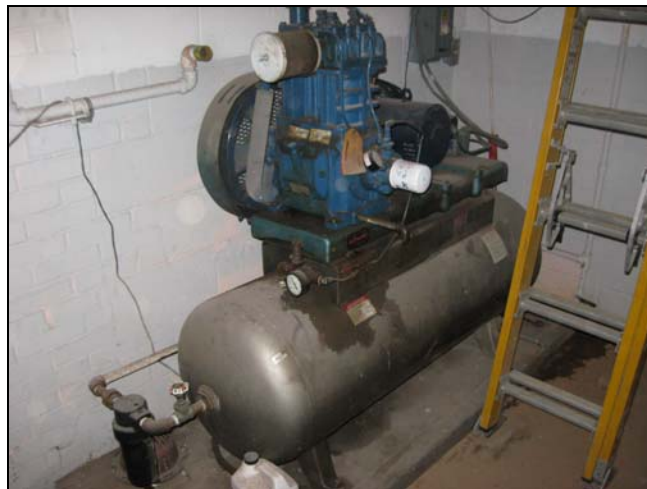
Air Compressor for Shop Area
