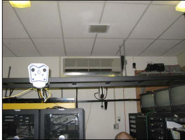
Indoor Section of Ductless Split System in IT Room
