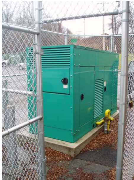
Figure E-5. Outdoor Emergency Generator
