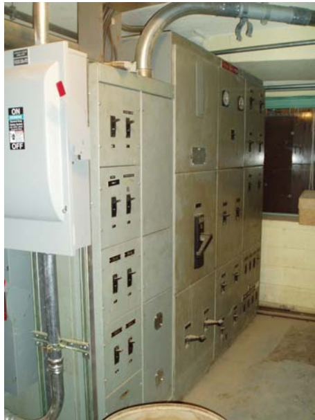
Figure E-2. Original Service Entrance Equipment
