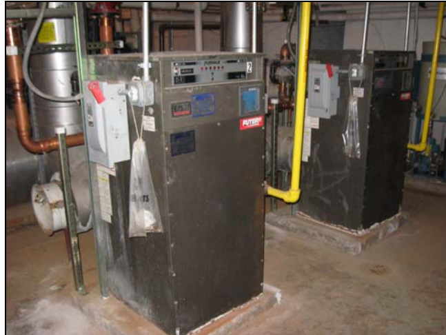
Boilers Used for Domestic Hot Water Generation
