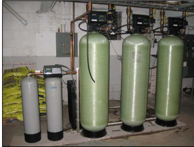
Water Softening System
