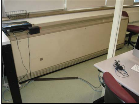
Typical Classroom Unit Ventilator
