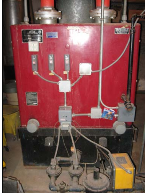
Boiler Used for Domestic Hot Water Generation
