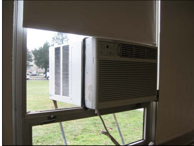
Window Air Conditioning Unit
