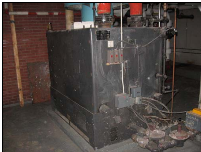
Boiler Used for Domestic Hot Water Generation
