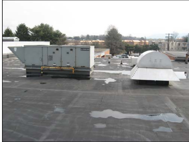
Kitchen Makeup Air Unit and Kitchen Hood Exhaust Fan
