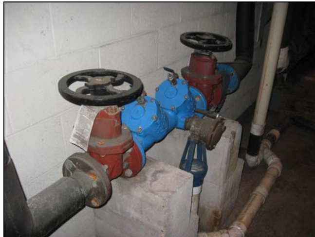
Backflow Preventer at Water Service Entrance
