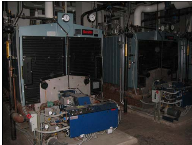
Two of the Three Heating Water Cast Iron Sectional Boilers
