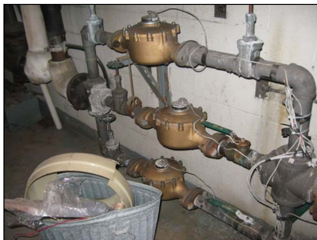
Domestic Water Meter Assembly at Water Service Entrance
