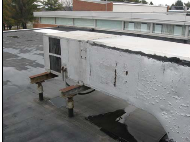
Packaged Rooftop Unit
