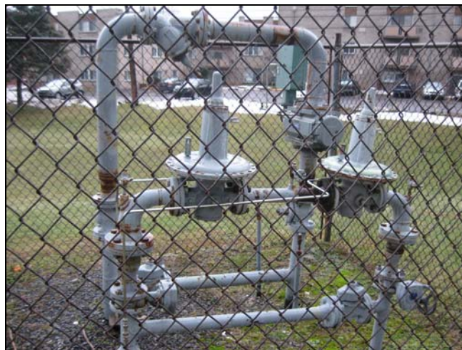
Natural Gas Service Entrance
