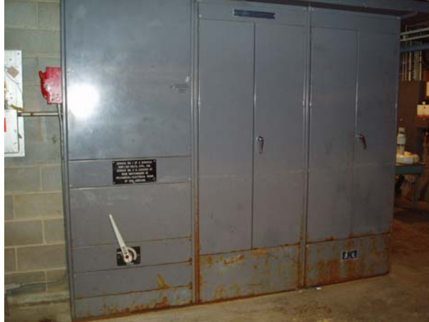
Figure E-1. Service Entrance Equipment One
