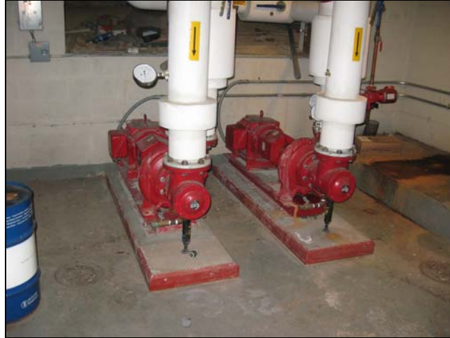
Heating Hot Water Circulation Pumps
