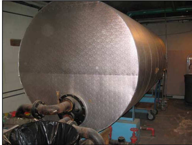
Domestic Hot Water Storage Tank
