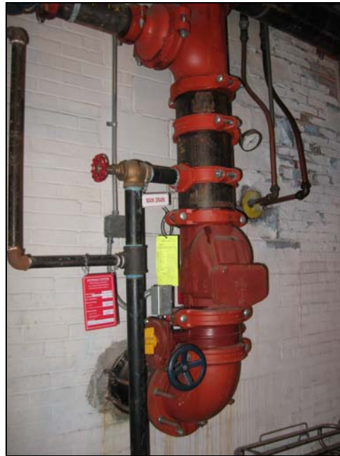
Sprinkler Water Service Entrance
