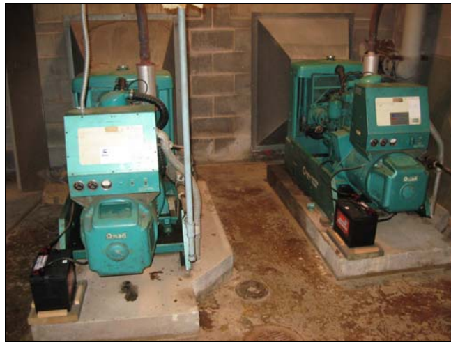
Figure E-3. Lower Level Generators
