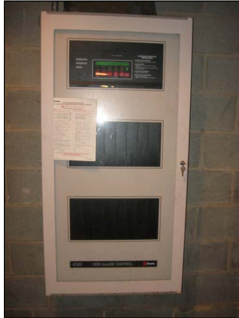
Fire Alarm Panel
