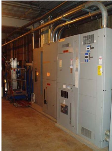
Figure E-2. Service Entrance Equipment Two
