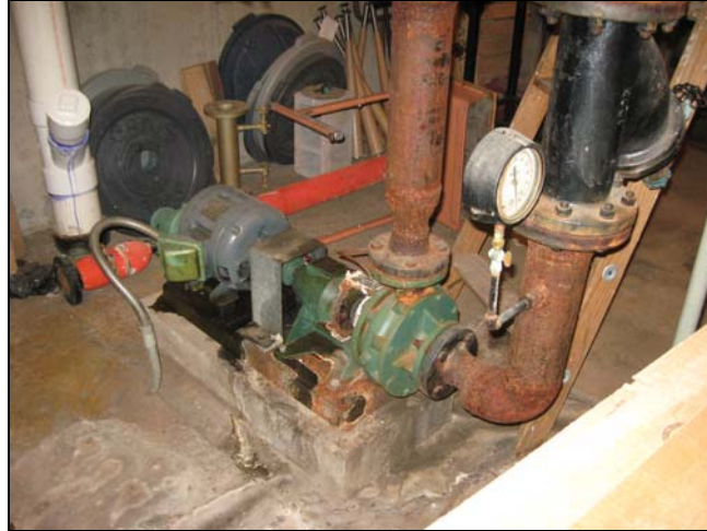
Chilled Water Pump
