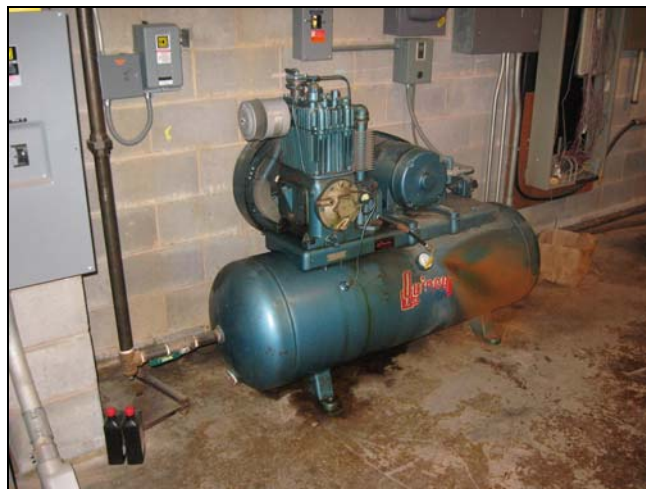
Air Compressor for Wood Shop
