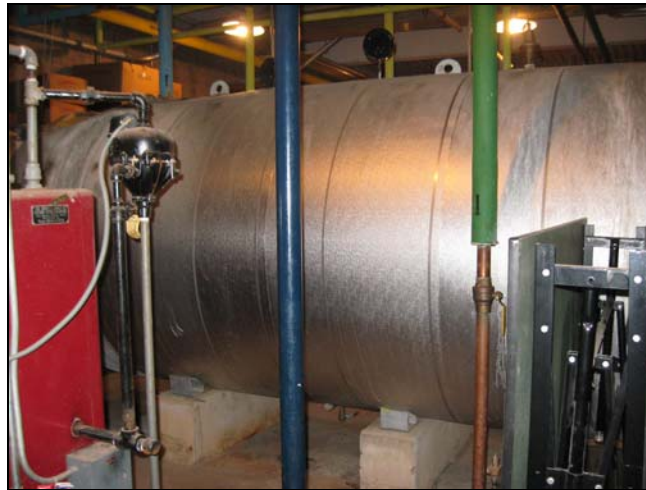
Domestic Hot Water Storage Tank
