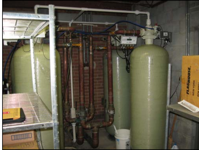
Water Softening System
