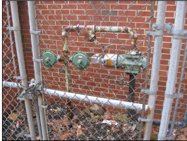
Natural Gas Service Entrance
