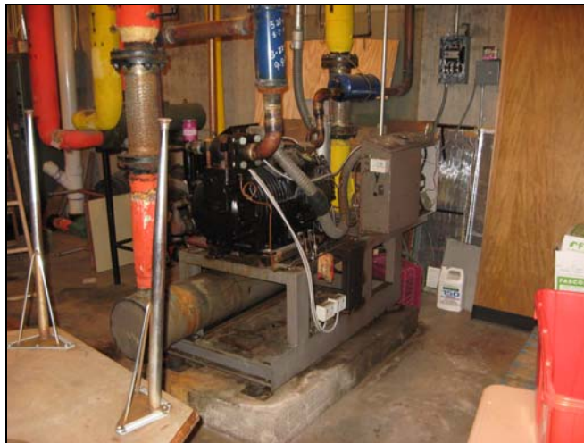
Indoor Section of Chiller
